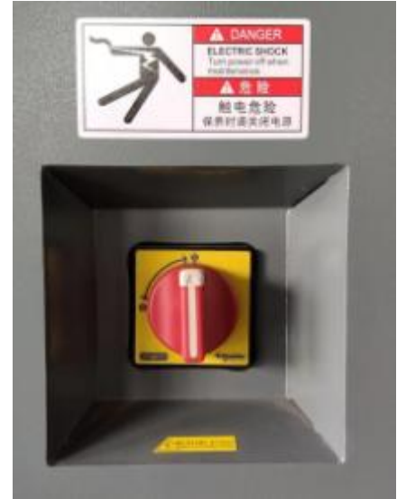
General power supply open status ON
