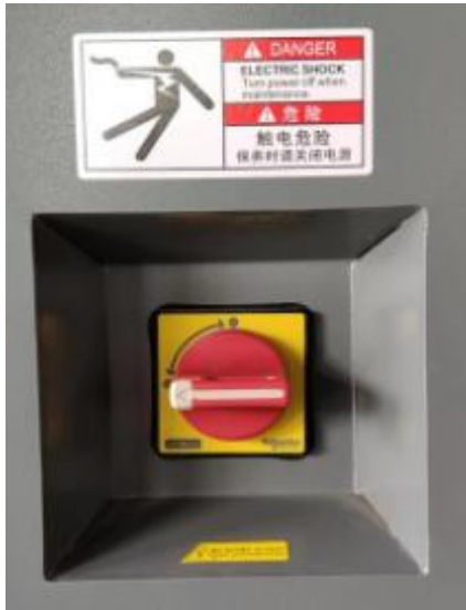
General power supply close status OFF
